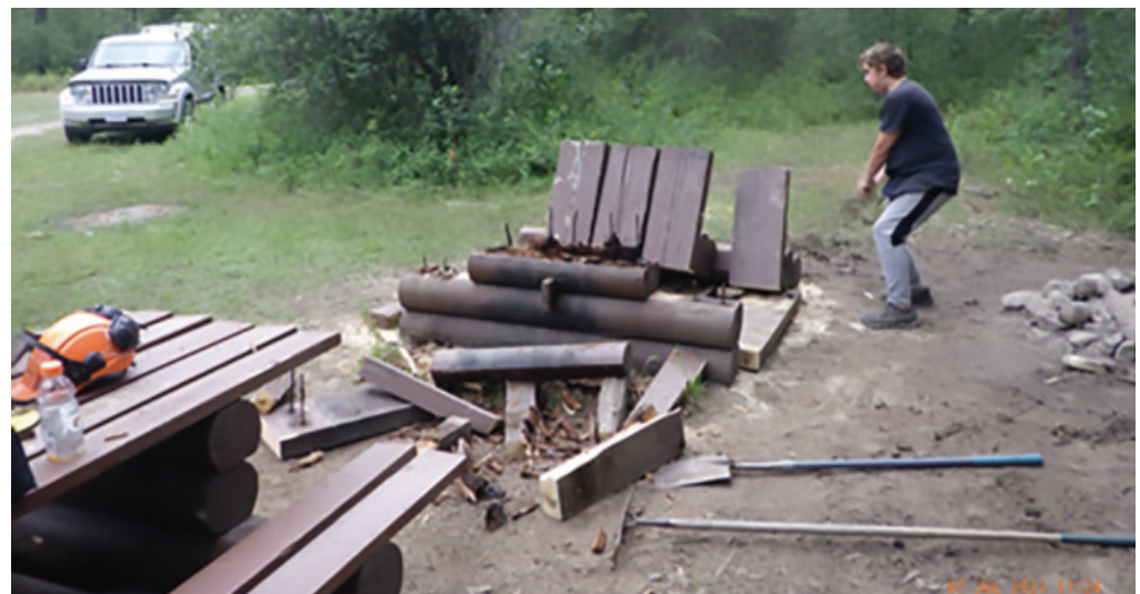
Out with the old and in with the new picnic table Work crew changing 3 picnic tables at Bluejoint Rec Site.
